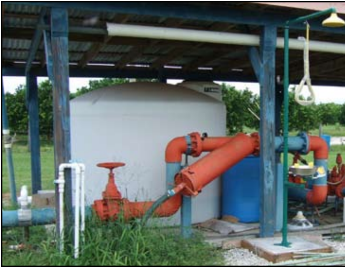
Fig. 6.3. Nutrient solution sources for fertigation are stored in large plastic tanks at the irrigation pump station. (Thomas Obreza)
